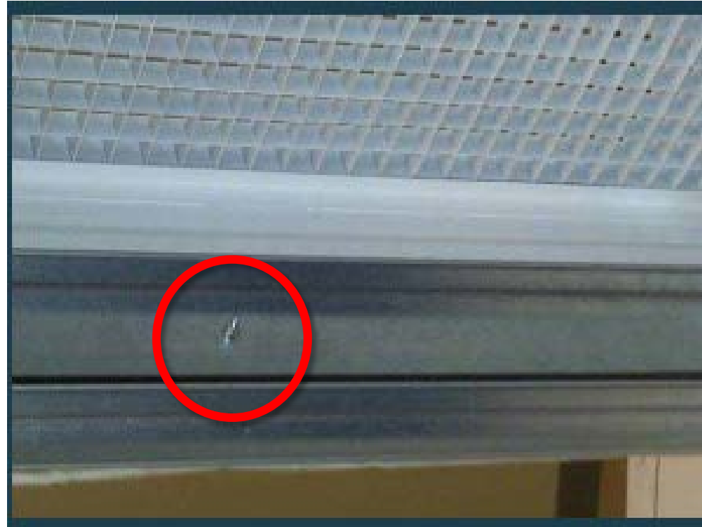
The installation screw is in the track of the damper
