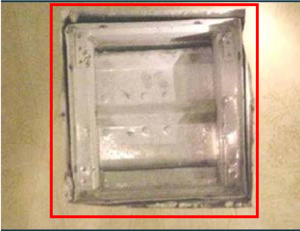
The damper is installed racked
