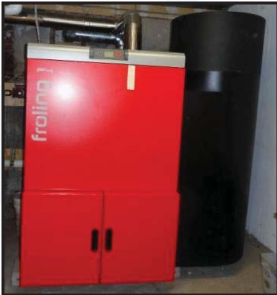
Frohling P4 Boiler
